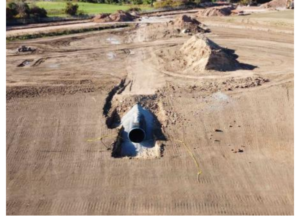
Retention pond storm water inlet (10/19/2021)
